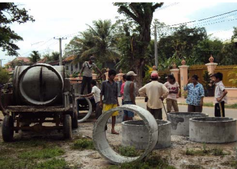
Mrs. Pen Sophea working with her Sanitation Self-Help Group to arrange for the transport of the toilet materials to the household construction sites Photo © UN-Habitat
